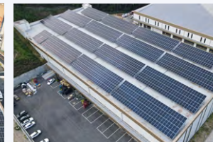
SK networks Icheon Distribution Center (self-consumption)
