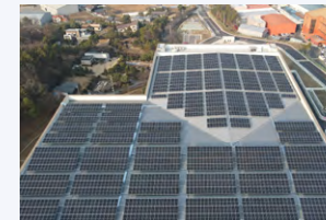
Solar Power Plant No. 1 (power generation business)
